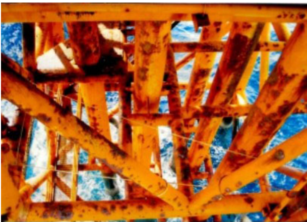
Fig. 1. Corroded platform BK-1 at White Tiger field (photo courtesy of VSP)
