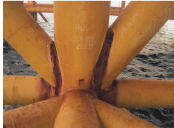
Fig. 2. A corroded tubular joint in platform MSP6 at White Tiger field (photo courtesy of VSP)
